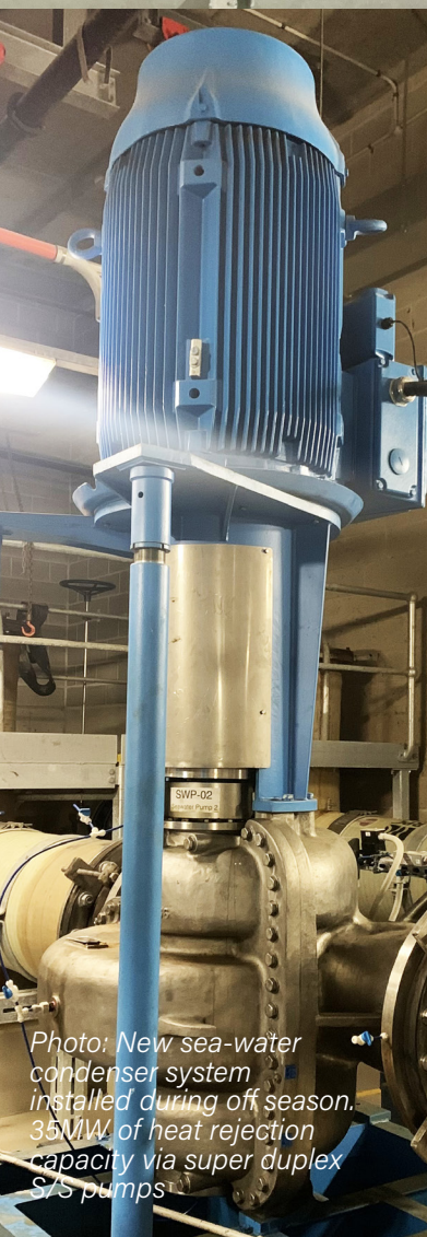
Photo: Primary CHW and CDW pumps for a 22MW Mechanical Central Energy Plant
